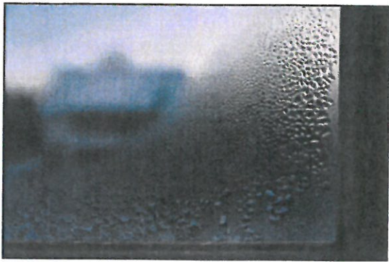
Condensation on the inside of a window-pane.
